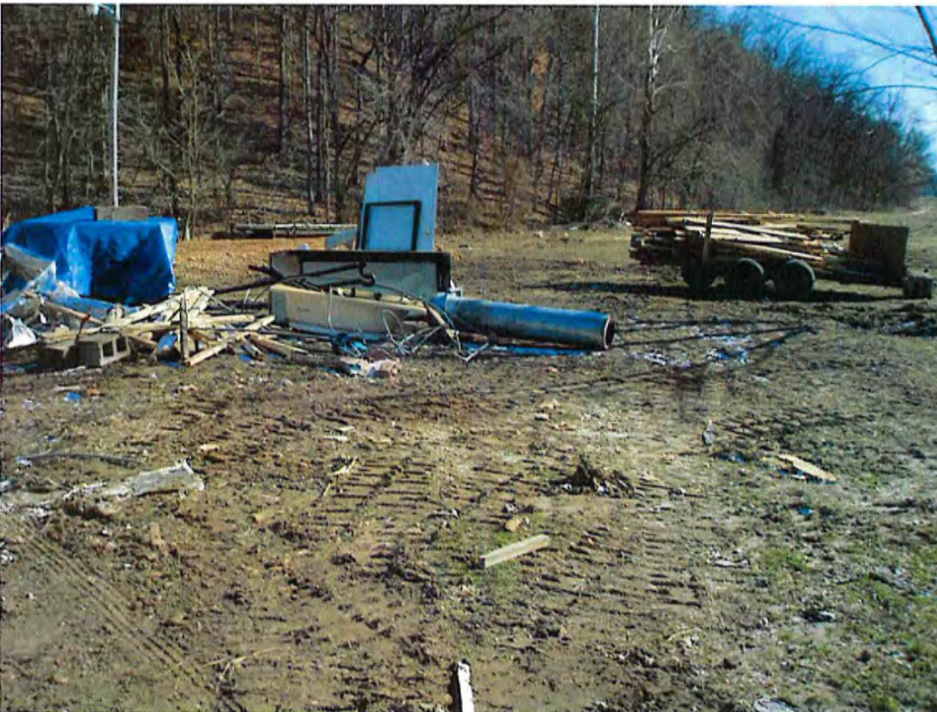
Date: 1/3/2014 Time: 1:09 P.M. Direction: southeast Photo by: S. Williams Exposure #: 018 Comments: trailer with wood on it, bathtub, a variety of metal, doors, and scattered demolition debris
