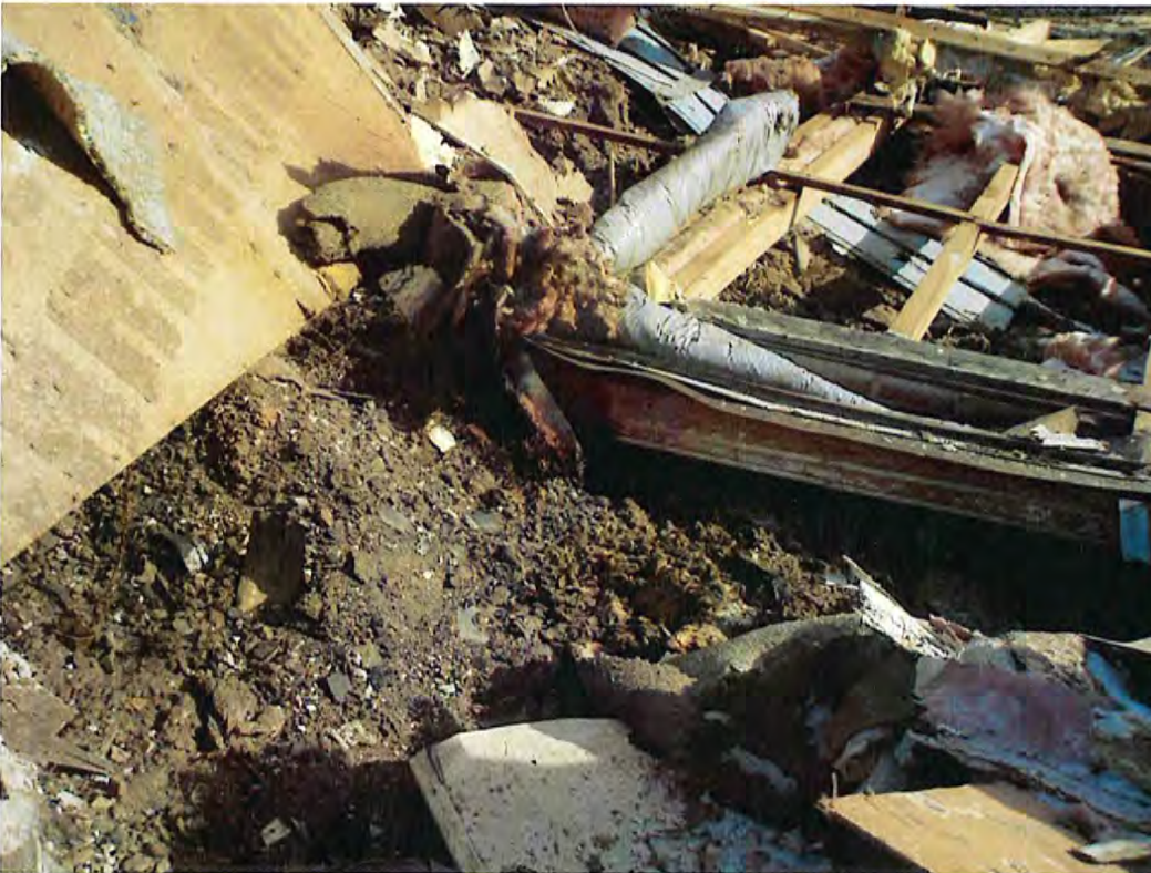
Date: 1/3/2014 Time: 12:46 P.M. Direction: east Photo by: S. Williams Exposure #: 008 Comments: smoke was observed wafting from demolition waste
