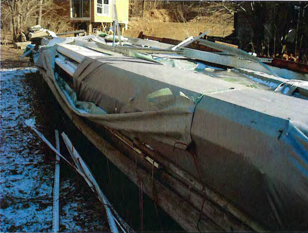
Date: 1/3/2014 Time: 1:03 P.M. Direction: southeast Photo by: S. Williams Exposure #: 017 Comments: shingles & siding on a trailer, partially covered by a tarp
