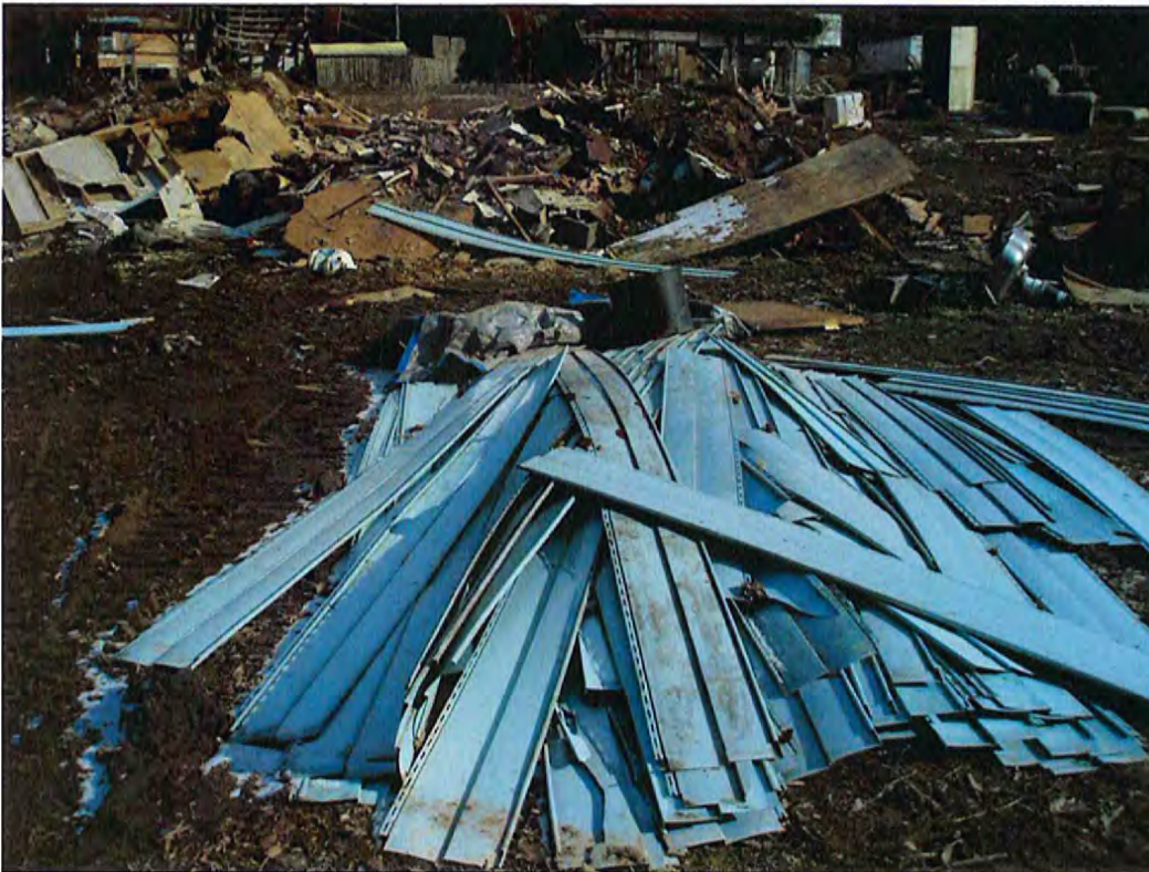
Date: 1/3/2014 Time: 12:50 P.M. Direction: east Photo by: S. Williams Exposure #: 010 Comments: variety of demolition debris
